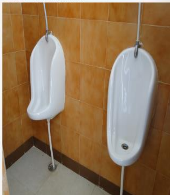
URINAL - TILED WASHROOM
